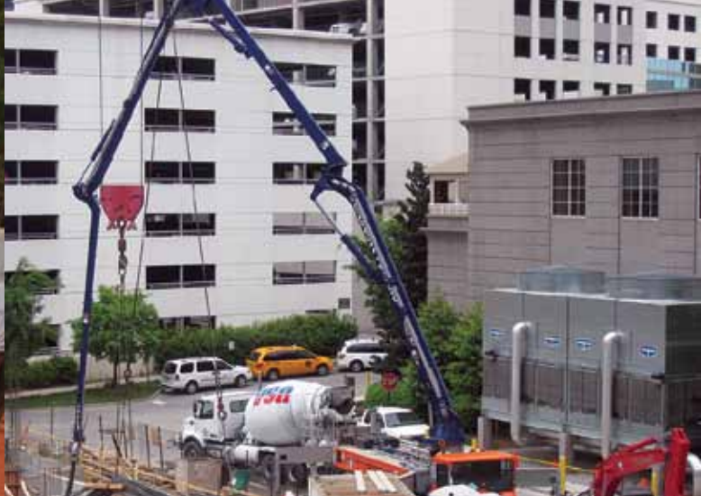
The S 36 provided the versatility needed on the Circle Terminus apartment project in Atlanta.
