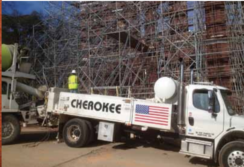
A recently acquired Schwing SPTO 2000 will pump the decks for the five stories of apartments that will be built over the parking structure.
