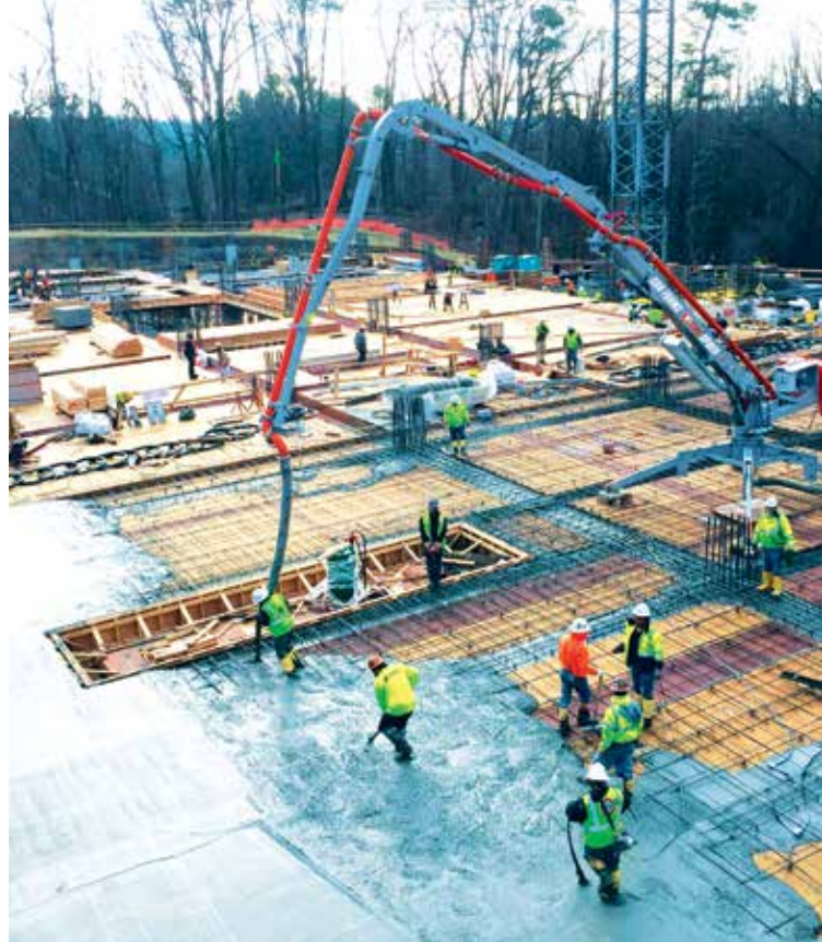
The boom is easily repositioned on the deck and plugged into the pump's end hose to take the place of a separate placing boom at less cost.
