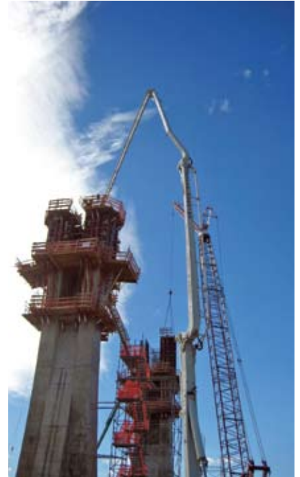
Forming and pouring of the splayed super columns occurred simultaneously in order to meet the May 1 deadline for track beam construction.
