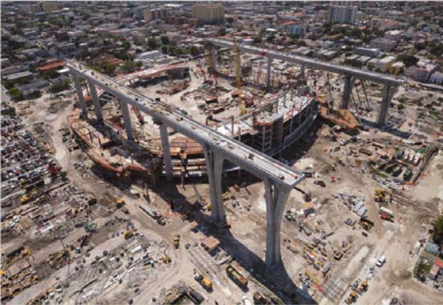
Splayed columns can be seen at the end of the track. Track beams were cast-in-place on the first section in order to speed construction while pre-cast beams were hoisted into position.
