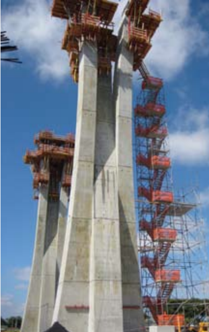
Jump forms were used to place 13-foot lifts which took up to a week to pour due to the shape and tight tolerances of the super columns.
