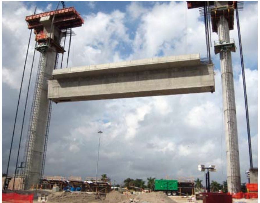
Hydraulic strand jack was used to lift precast track beam sections that were pumped at the lifting point.
