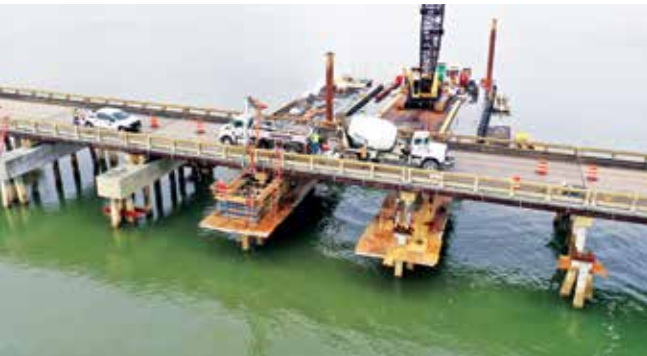
Excessive scouring from recent storms made the addition of piles—shown here in the foreground of each bent—necessary to improve the structural integrity of the bridge. Once installed, they were capped with the 71-cubic-yard structure.
