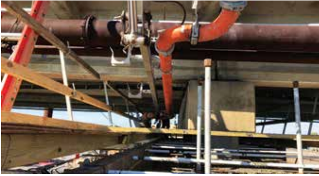
Cherokee CP's inability to pump over traffic made the addition of slickline beneath the bridge deck necessary to reach some of the farthest parts of the pour.
