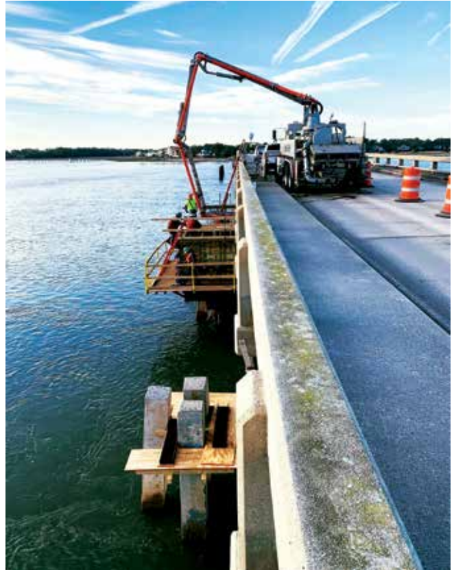
Being able to pump directly off the side of the bridge to the piers below, rather than barging in equipment and personnel for the pours, helped keep production levels up on the Fripp Bridge retrofit.
