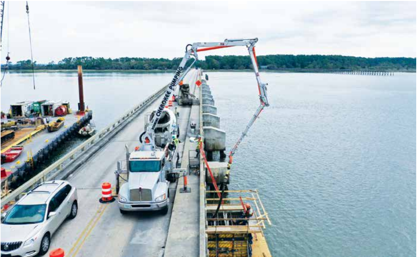
The compact design of the Schwing S 20 pump's outriggers allowed the pumper to work while traffic flowed freely in the remaining open lane of the 1,900-foot Fripp Inlet Bridge.
